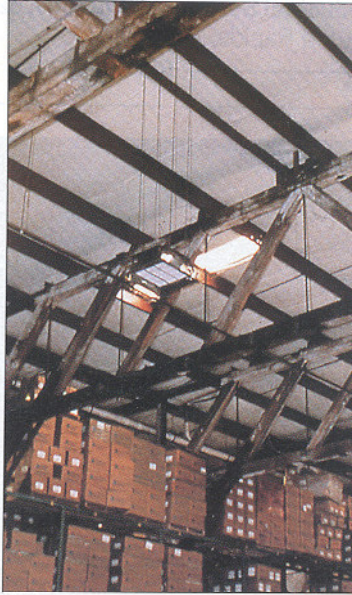
Installed on the warehouse ceiling and directed at the loading dock, the UET-120 ultrasonic device has eliminated a serious problem with bird droppings for Wheaton Injection Molding Co.
